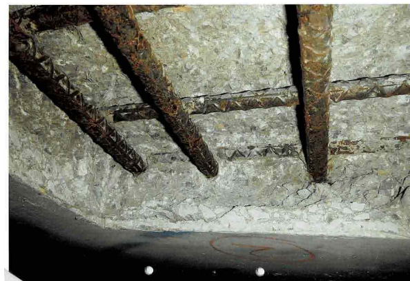
Figure 6: State of deterioration on the bottom surface of concrete slab
