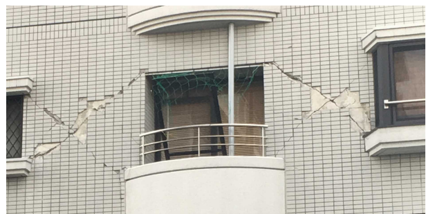
Figure 1: An example of a damaged non-structural wall in the 2016 Kumamoto earthquake
