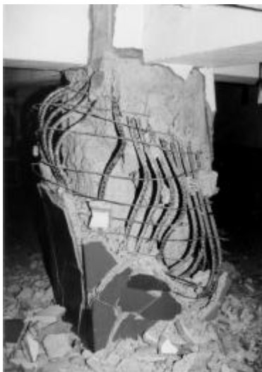
(a) Collapse due to shear failure of columns
