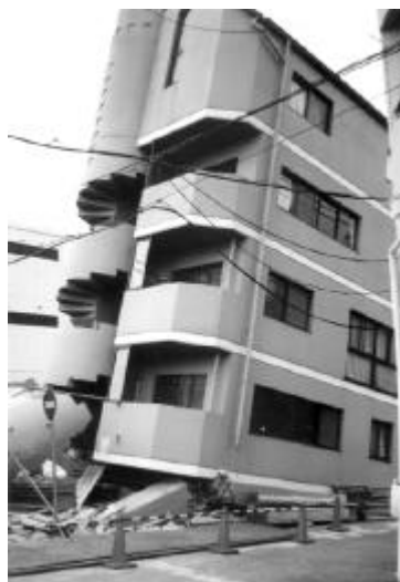
(b) Collapse due to excessive drift of the soft-first story
