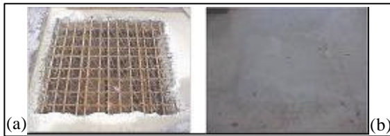
Figure 2. (a) Damaged concrete removed by a high-pressure water jet (hydro demolition) (b) repaired slab.
