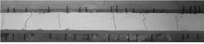
Figure 11. Primary cracks in the test employing the round bar at age of 0.5 days
