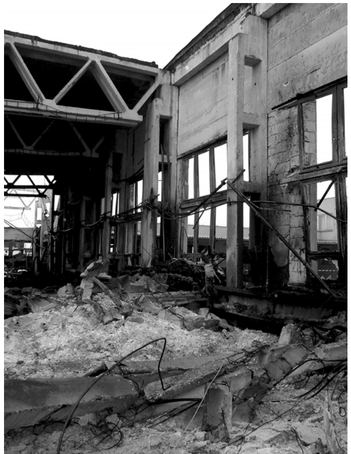
Figure 2. A collapse of joining balks and membrane roofing.
