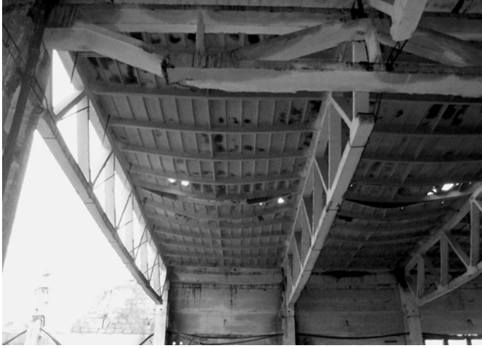
Figure 3. Local places with totally burned through membrane roofing.
