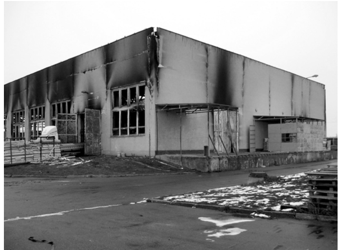
Figure 1. Fire affected hall.
