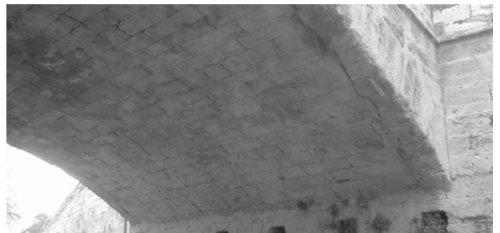
Figure 1. Damage in the stone in the end bridge bays.
