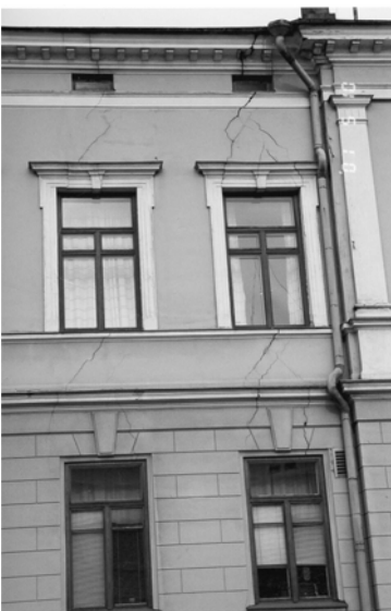
Figure 2. This kind of cracks in facade are usually a sign for uneven settling of the building foundations.
