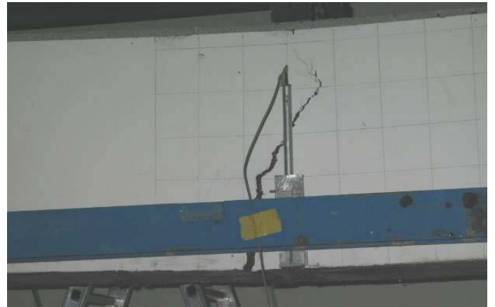
Figure 18. R/C HPFRCC jacketed beam: localization of the main crack.
