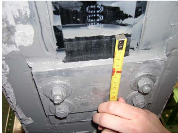
Figure 10. Failure of end anchorage (beam RC-EA).
