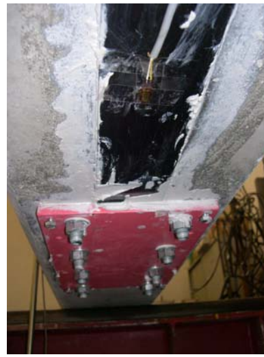
Figure 8. Steel bolted plate anchorage for RC-PrEA and PRC-PrEA beams.
