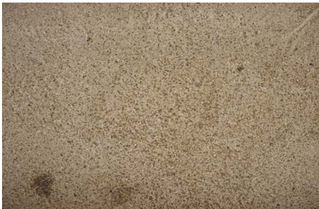
Figure 33. Surface of fire protection coating after test.
