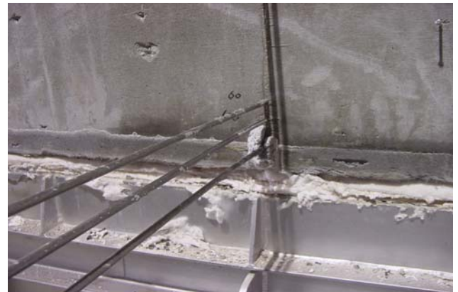
Figure 40. Water steam stain at the interface.
