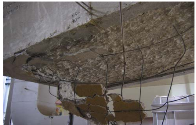
Figure 25. Separated fire protection coating.
