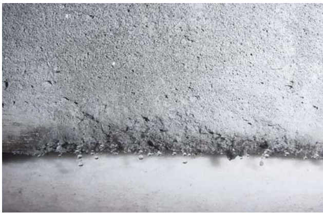
Figure 32. Water drops formed on the fire protection coating.
