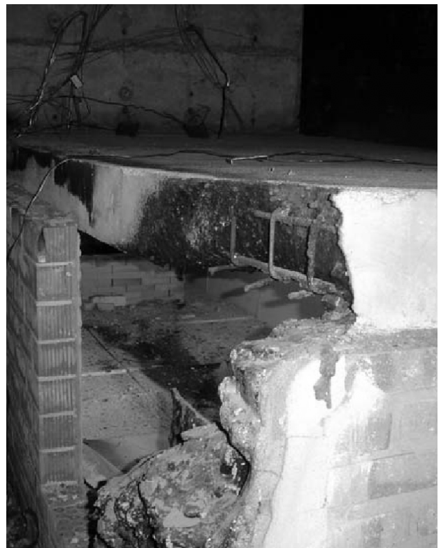
Figure 15. Photo from the experiment showing an extensive damage at the ceiling corners.
