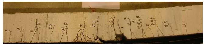
Figure 4. Final crack pattern for the beam C2-M033-L2.
