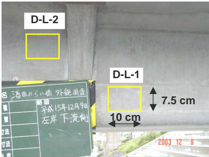
Photograph 5. Aesthetic observation masking of D-L-2 and D-L-1 on downstream side.
