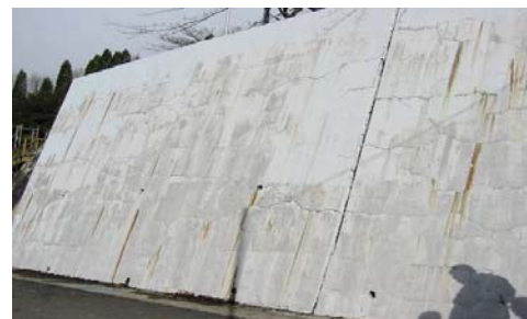
Figure 1. ASR-cracked concrete retaining wall.
