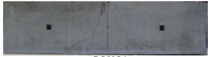
Figure 10. Crack pattern of RO80O4.
