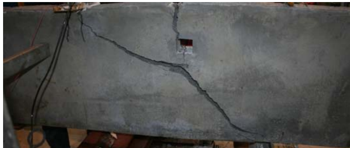
Figure 5. Crack pattern of RO80U3.
