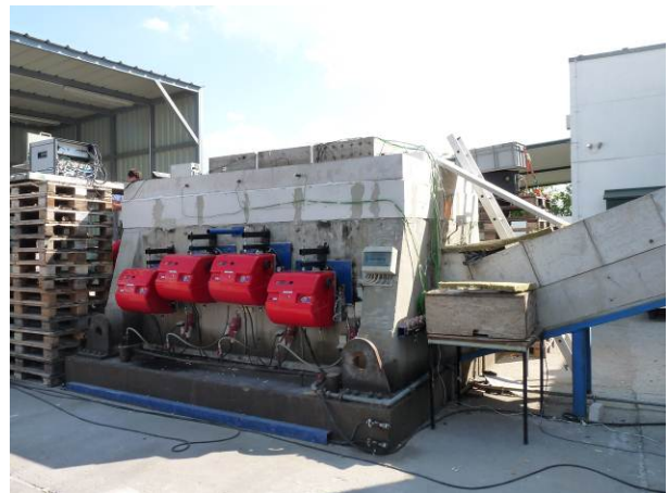
Figure 3: Furnace with four burners on both sides.
