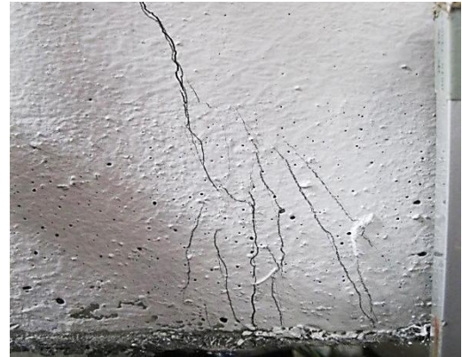
Fig 8 : Crack diffusion behavior in beam BREC-T
