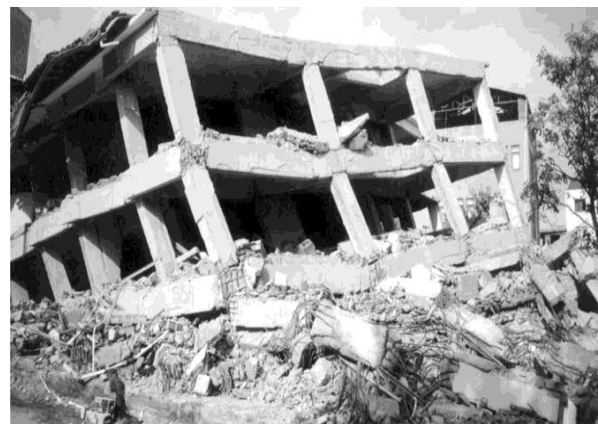
Figure 1: Beam-column joint shear failure in RC buildings [1].
