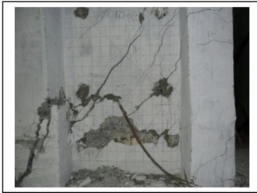
Figure 10: Spalling of concrete on compression flange and bottom portion of web wall in RSW-MO-1.25.
