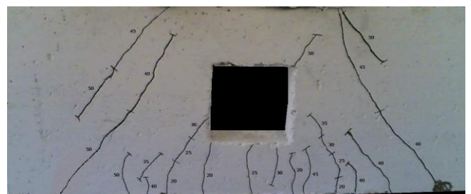
Fig. 20. Crack pattern and mode of failure of beam BOC3 (4Ø12 CFRP) ( P_{cr} = 200 KN and P_{ult} = 500 KN)
