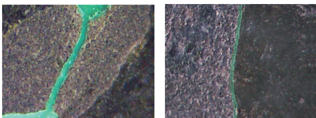
Figure 3: Enlarged view of epoxy impregnated cracks within the matrix phase (left) and along the matrix-aggregate interface (right)
