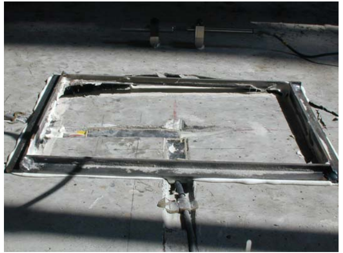
Figure 14. Punching shear failure. Zone N3N4. Top side.
