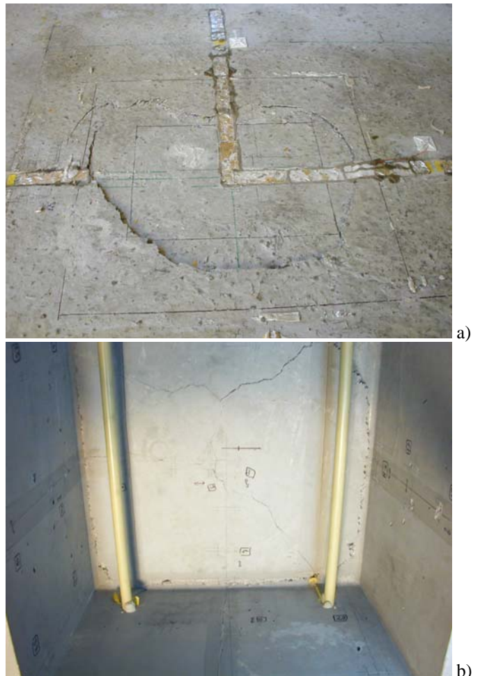
Figure 15. Punching shear failure. Zone N2N3. a) Top side. b) Bottom side.
