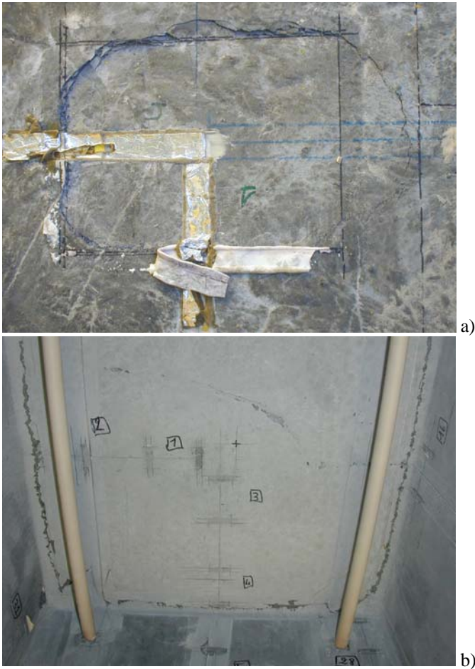
Figure 16. Punching shear failure. Zone N6N7. a) Top side. b) Bottom side.
