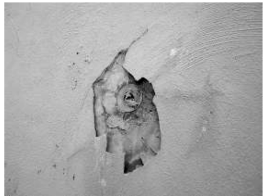
Figure 10. Typical place with left formwork spacer. Water leaks and concrete degrades near the spacer and spacer sealing area.
