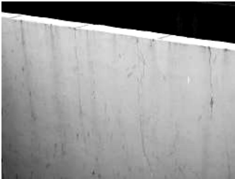
Figure 4. Front face of discharge conduit construction. Vertical cracks from the top to the bottom.
