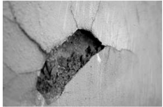
Figure 9. Detail of degraded repair mortar.
