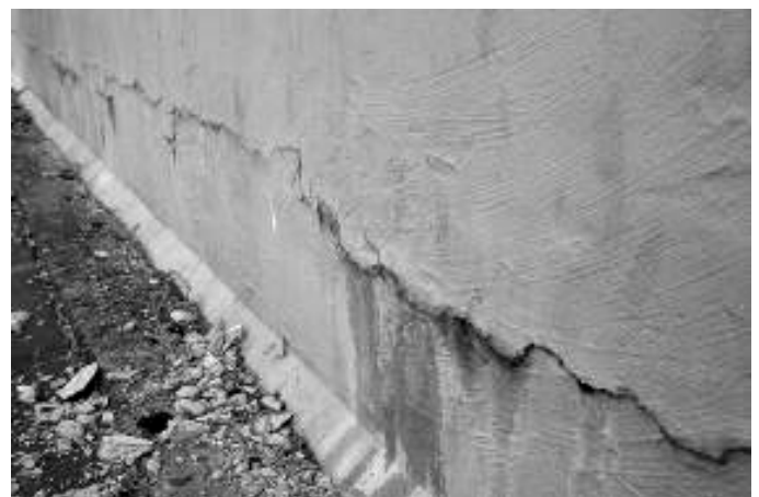
Figure 2. Front face of discharge conduit construction. Detail of crack between foundation and construction of discharge conduit.
