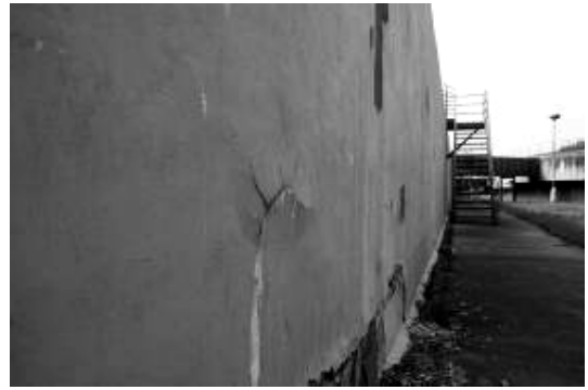
Figure 8. Typical separation of renovation plaster on the front wall of the conduit.
