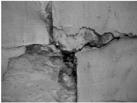
Figure 3. Surface of the wall structure No. 1, external surface. Crack near the dilatation joint, connection of foundations and conduit structure.
